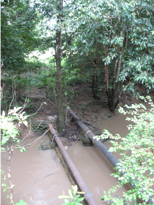
Photo L.1 PROPOSED NORTHERN CROSSING POINT AT SIX MILE CREEK (LEFT BRANCH) LOOKING EAST
